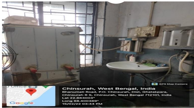
Water purifier of Zoology Dept with water cooler
